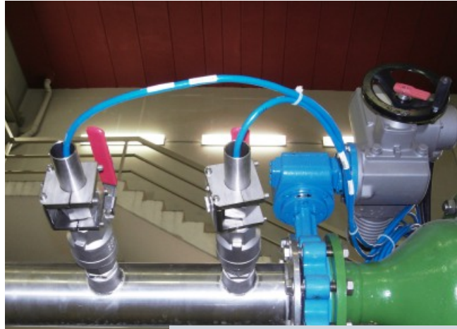
Nighttime supply flow measurement single path measurement in a full filled pipe
