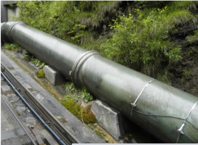
Turbine intake flow measurement using clamp-on sensors
